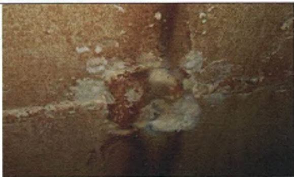
Apparent pit repair on interior sidewall seam
