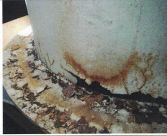
Stiffener on wet interior access tube
