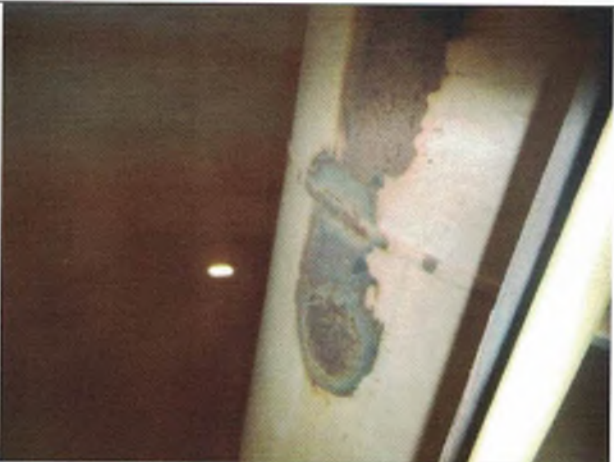
Wet interior access tube
