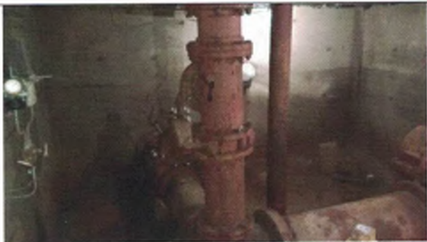
Piping in lower level of pump house
