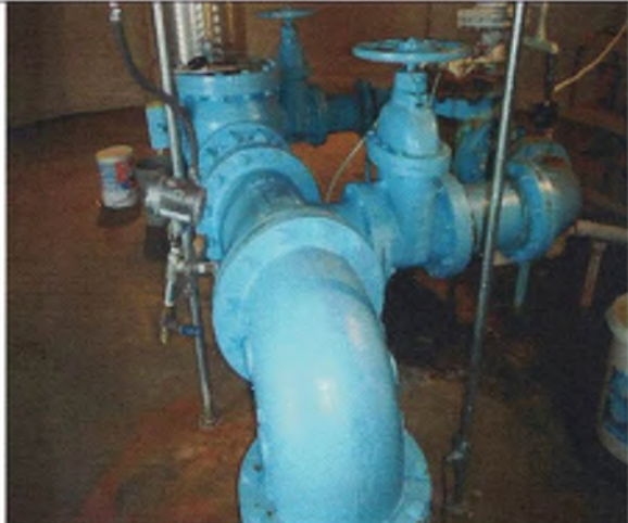
Pipes in basebell
