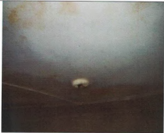
Wet interior roof
