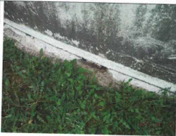
Spalling of foundation
