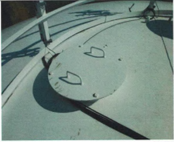
Secondary roof hatch cover
