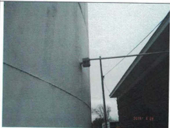
Conduit for cathodic protection entering the north sidewall
