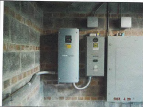
Controls in pump house
