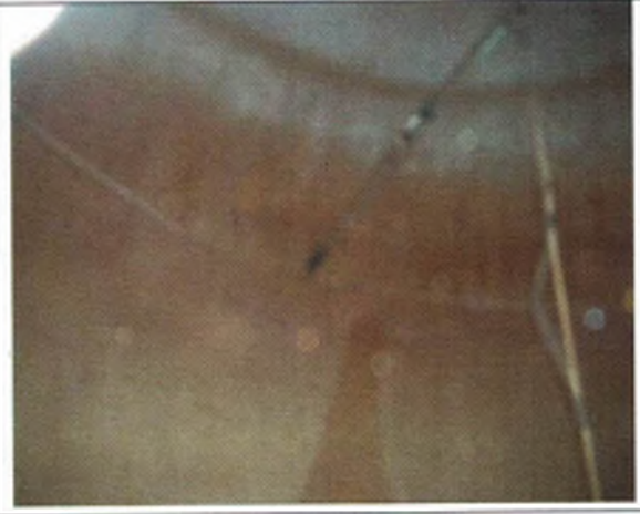
Cathodic protection and equator
