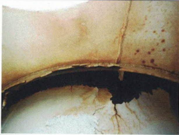
Wet interior access tube and roof
