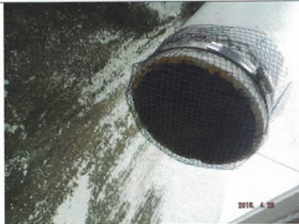
Overflow pipe screen
