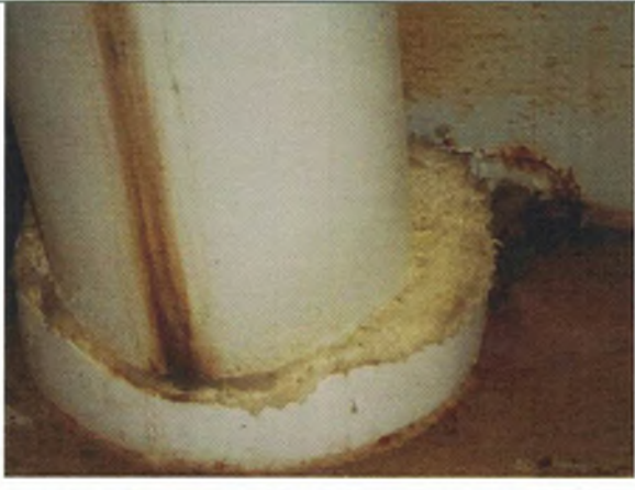
Overflow pipe in condensate platform
