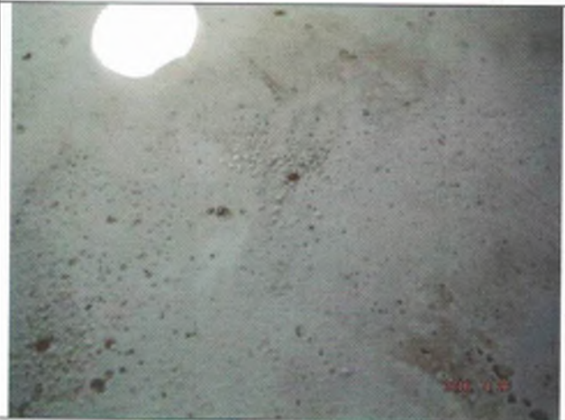
More blistering of coating on floor
