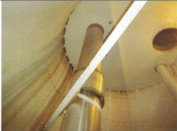
Fill pipe; staining on upper basebell wall
