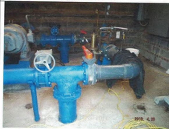
Piping on main floor of pump house
