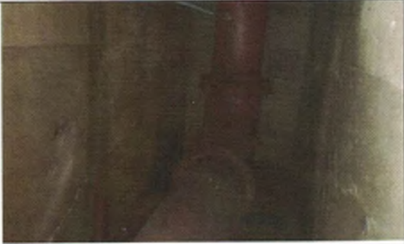
Fill line in lower pump house
