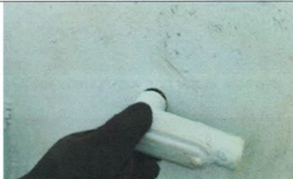
Obsolete conduit entering tank roof is loose
