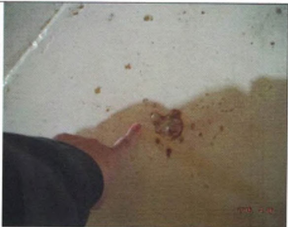
Blistering of coating on floor
