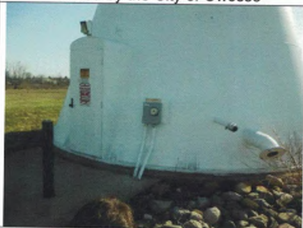
Basebell door and pipes
