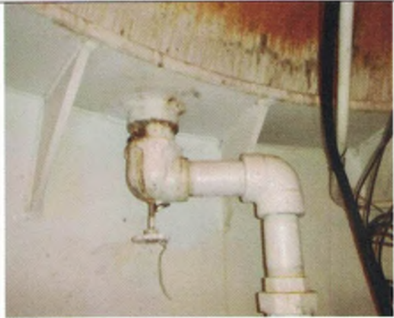
Mud valve under the inverted cone
